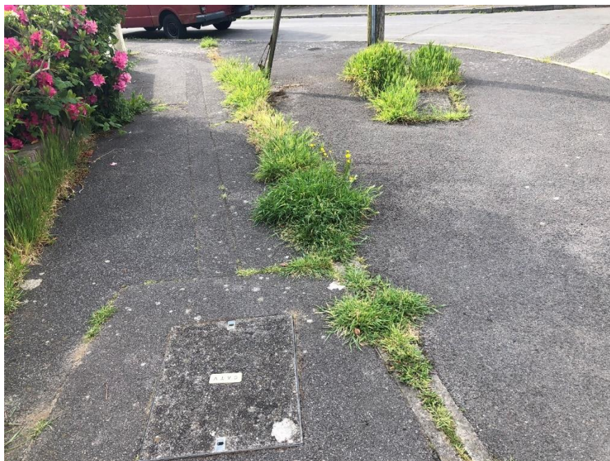
Fig. 2 [Weed Growth in Drainage Channel]
