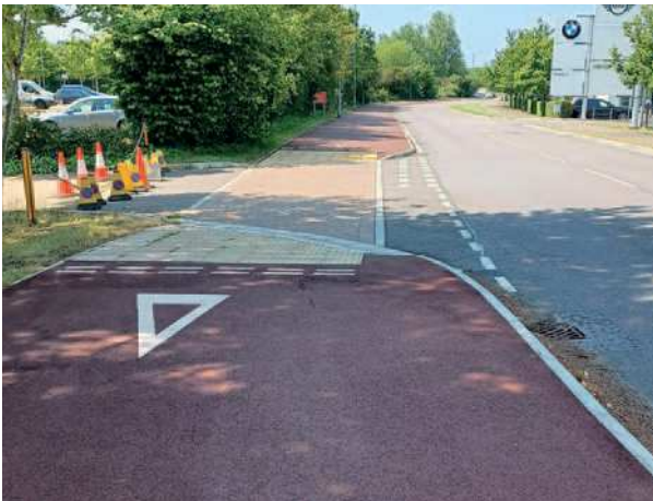
Photo 21: Priority given to vehicles accessing car park rather than those using the shared path, (note: in this urban location cyclists and pedestrians should also be segregated) Cambourne, South Cambridgeshire.
