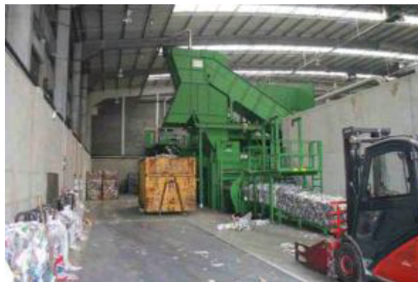
Bulking up facilities within a MRF
