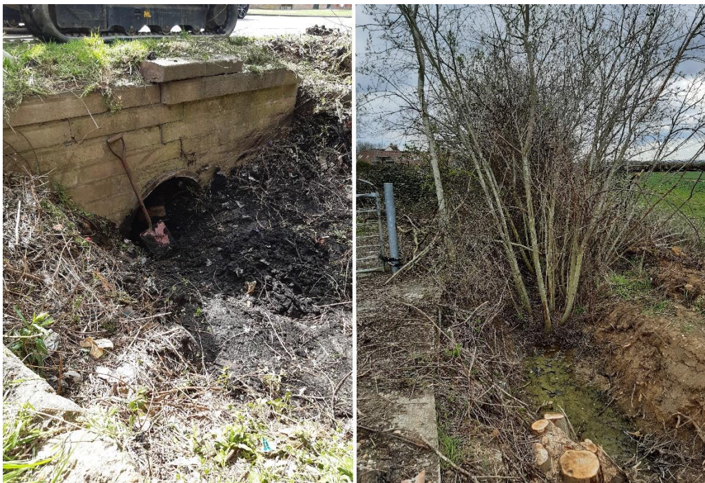
Figure 16: Examples of flow restrictions found through Section 19 investigations (2021)
