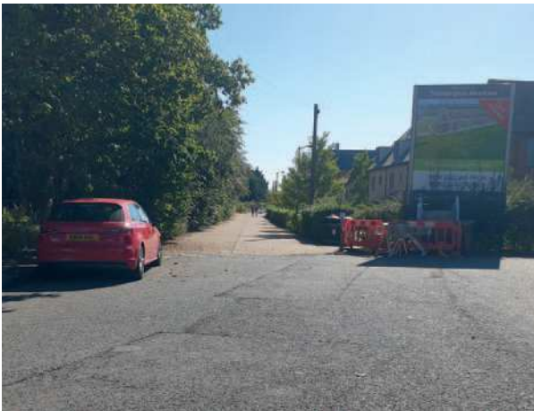
Photo 11: Poor provision for active travel connection between the existing supermarket and new development, Trumpington Meadows, Cambridge.
